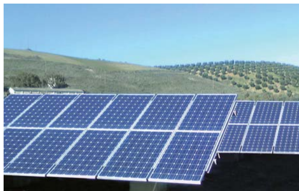
Solar power plant constructed in southern Italy
