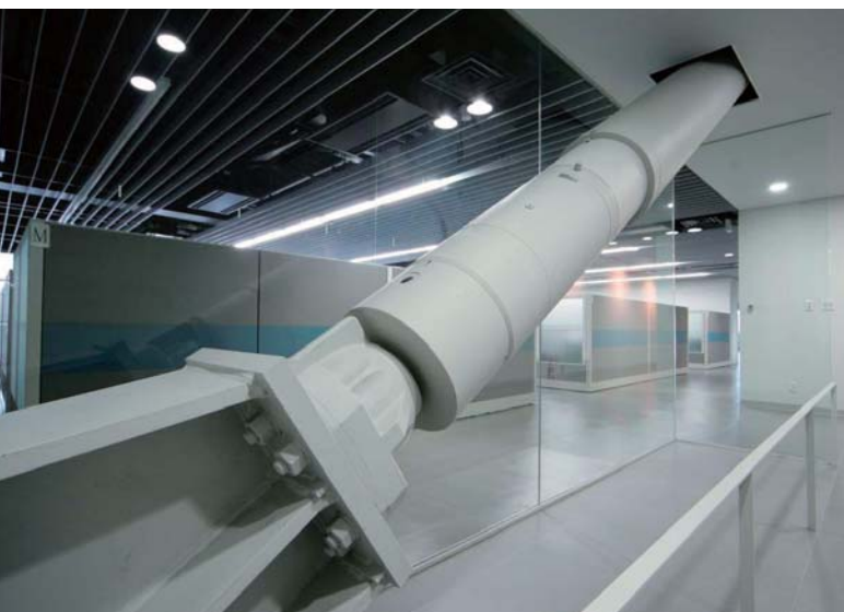
There are approximately 570 seismic dampers inside the plant for absorbing earthquake vibrations
